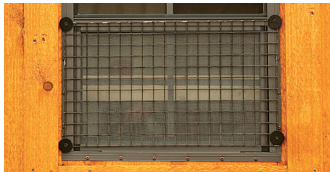
Wire over window
